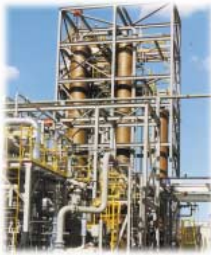
Water treatment skid for modular plant design.
